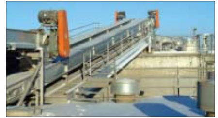
Two Schlagel 15,000-bph drag conveyors that carry grain out to the new slipform concrete annex.
