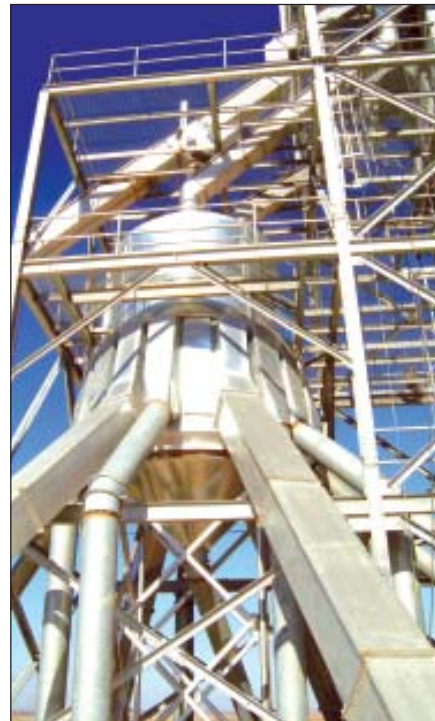
New 22-duct, Schlagel electronic programmable triple distributor handles the output of three legs at once and can keep three different commodities separate simultaneously.
