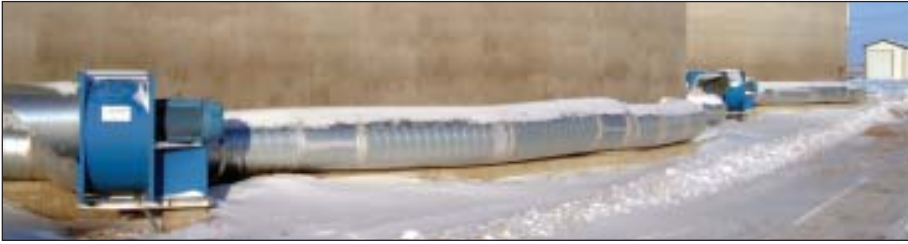
Airlanco centrifugal fans and ducting serving the PM Luft/KanalSystem floors in the new tanks.
