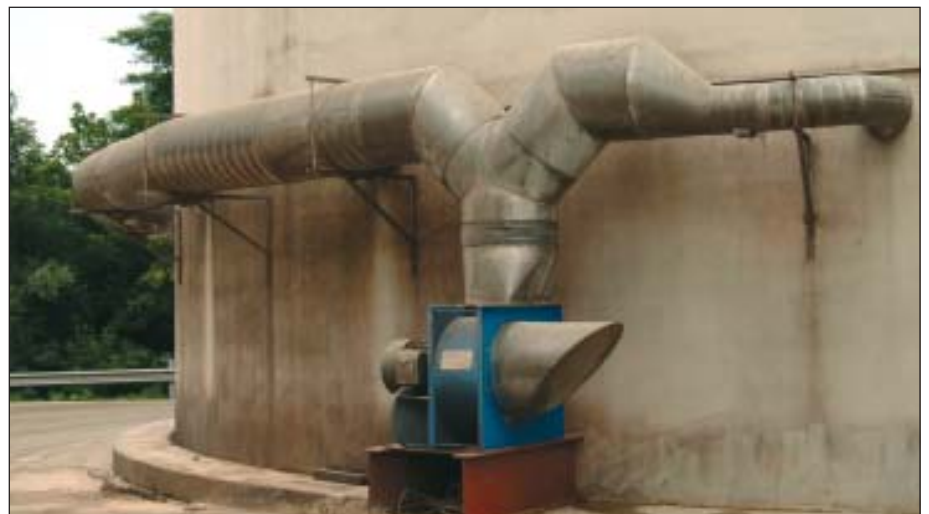
KanalSystem unit on the new tank provides air assist for unloading, although Pilgrim's Pride does not aerate grain in the tank.
