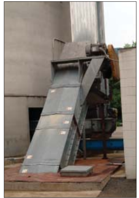
Inclined Essmueller drag conveyor deposits incoming corn into the boot section of the new Essmueller leg.
